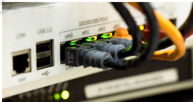
Figure 10.12: Cables connected to a network switch
